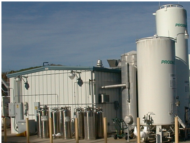
FIG. 1. Outside of the Hall B gas shed, showing argon and carbon dioxide dewars.
